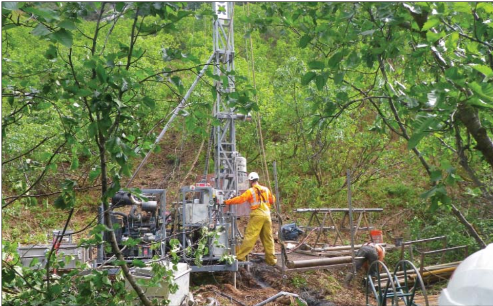
Left, contractor crews performing boring tests to help determine the geological conditions of the project site
