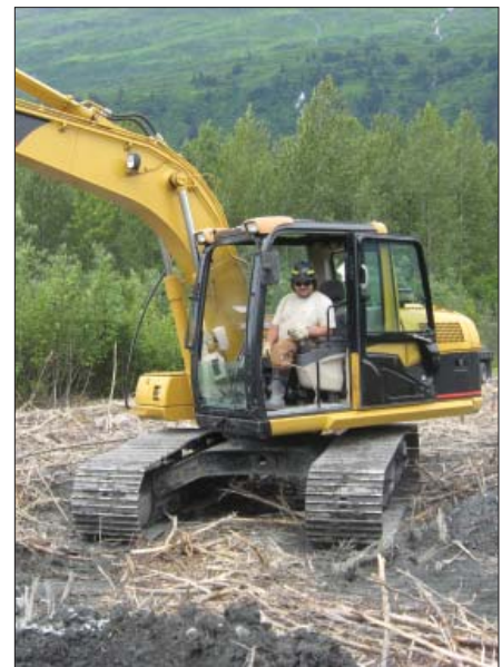
Top, KB Energy, LLC President Keith Broyles (left) and lead installer Terry Broyles (right) assisting CVEA during the installation of the MET tower.
