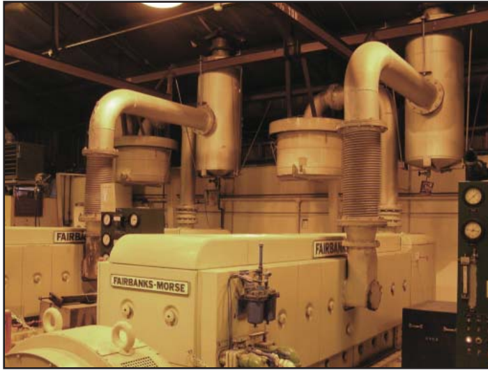
These Glennallen diesel plant dinosaurs, installed in 1959, will be replaced with a newer, more efficient engine in 2008.
