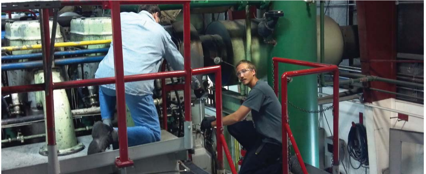
Terry DeLay, CVEA Valdez Plant Operator for over 20 years instructs Kyle Anderson, Valdez Plant Operator Trainee, on lock out/tag out techniques at the Valdez Diesel Plant.
