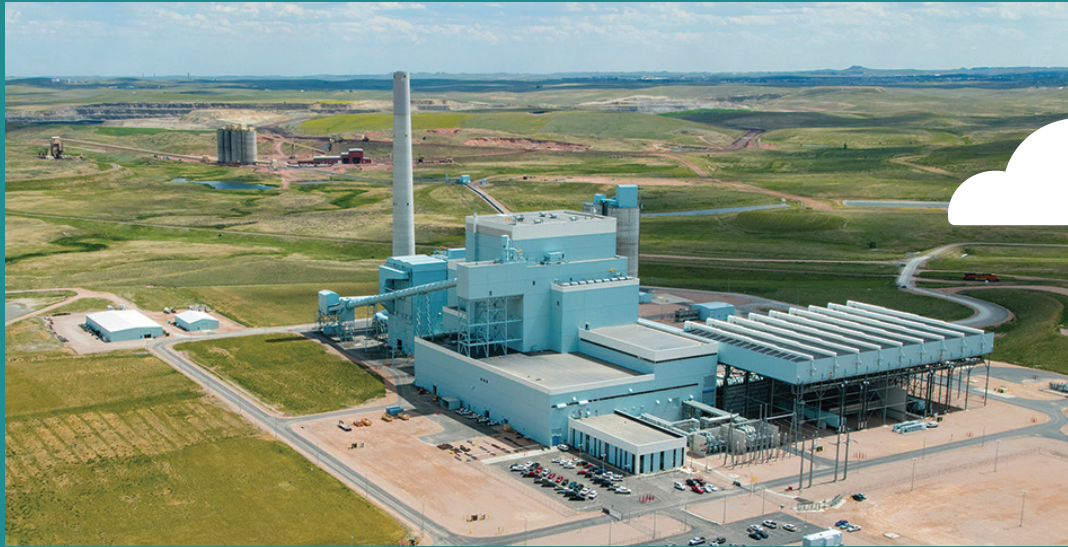
Basin Electric Cooperative's Dry Fork Station in Wyoming is near a site being developed for a large-scale carbon storage project.
